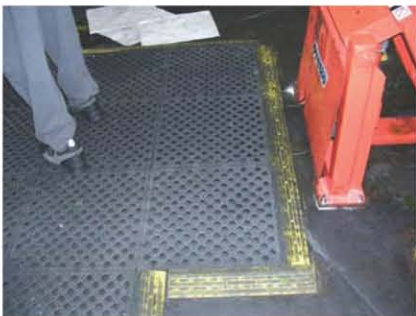
Electrical Cables run under mat
